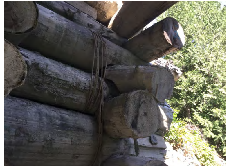
Tieback end sheared off upstream right bank
